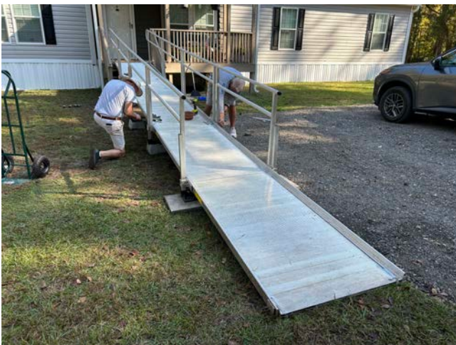
Community Service Project: PGK Ron Warner, Brother Gregg Koehn, Brother Joe Pourciau, and DGK John Molley installed a handicap ramp for parishioner Bill Cassell
